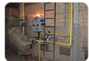
Floor space in Plant 2 was limited, so the new control panel was nestled alongside the kiln.
