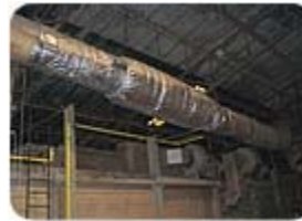
The ductwork in Plant 2. The expanded section is the "Torpedo."
